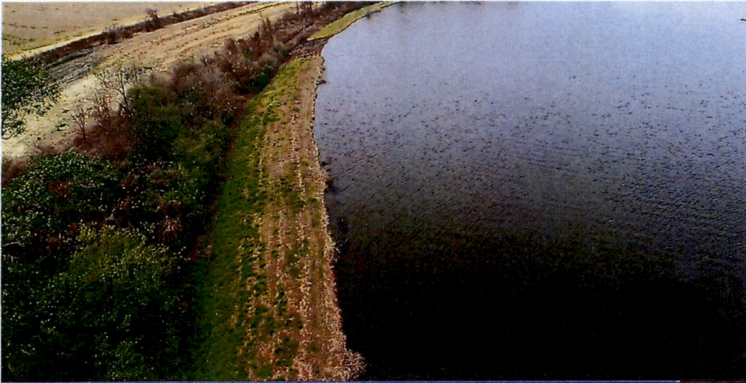
Photo 2. Helena WWTP South Wall Cell 3 Showing whole top of levee is gone
