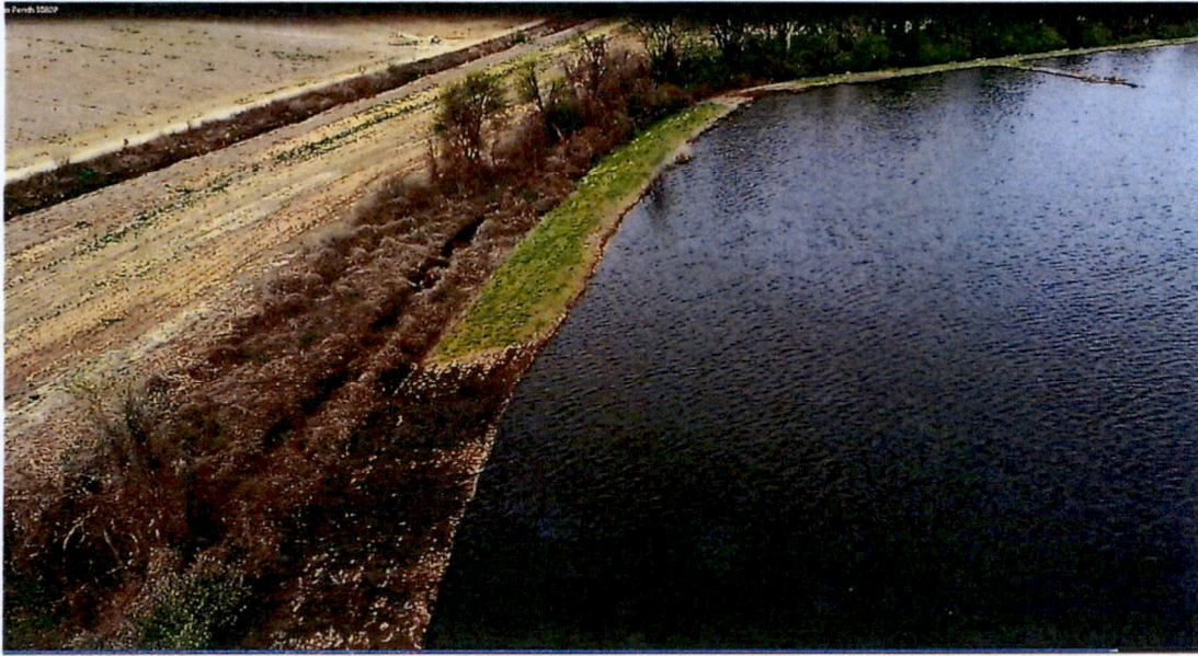
Photo 3. Helena WWTP Cell 3 South Wall Frontal View of Deterioration
